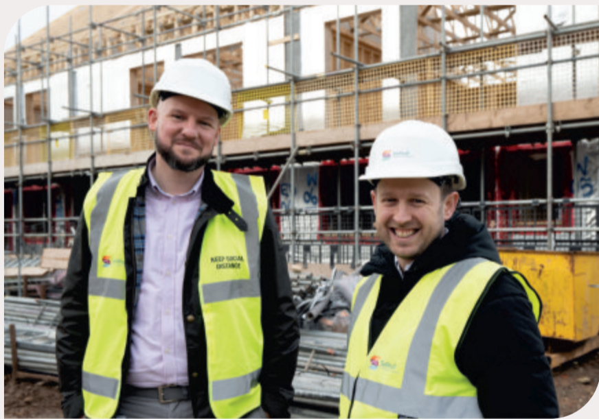
■ Head of Asset Management Andy and Development Officer Greg check out the build progress.
